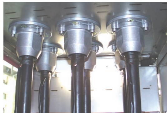
Fig. 6.5.1.1: View into the cable termination compartment in air with cable plugs and cables
